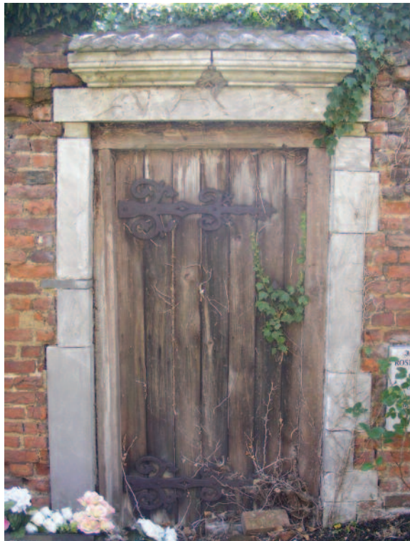
FIGURE 1 Doorway in the churchyard wall at St Michael's church, Horton, general view (Photo, author)
