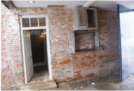
FIGURE 21 Carriage arch showing blocked original doorway to parlour G5 and meat safe
