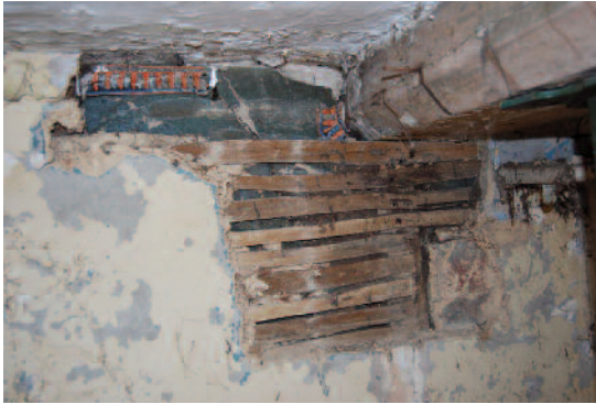
FIGURE 27 Remains of 1790s wallpaper in parlour G1
