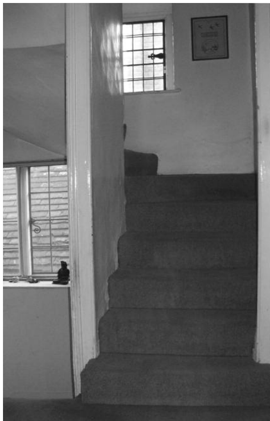
FIGURE 13 The 'winder' stairs between the first and second floors of Shell House (photo: Michael Rice)
