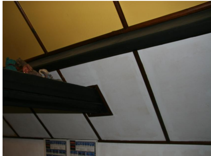
Figure 10: The curious position of the cross-beam in the study: below and separate from the roof purlins.
