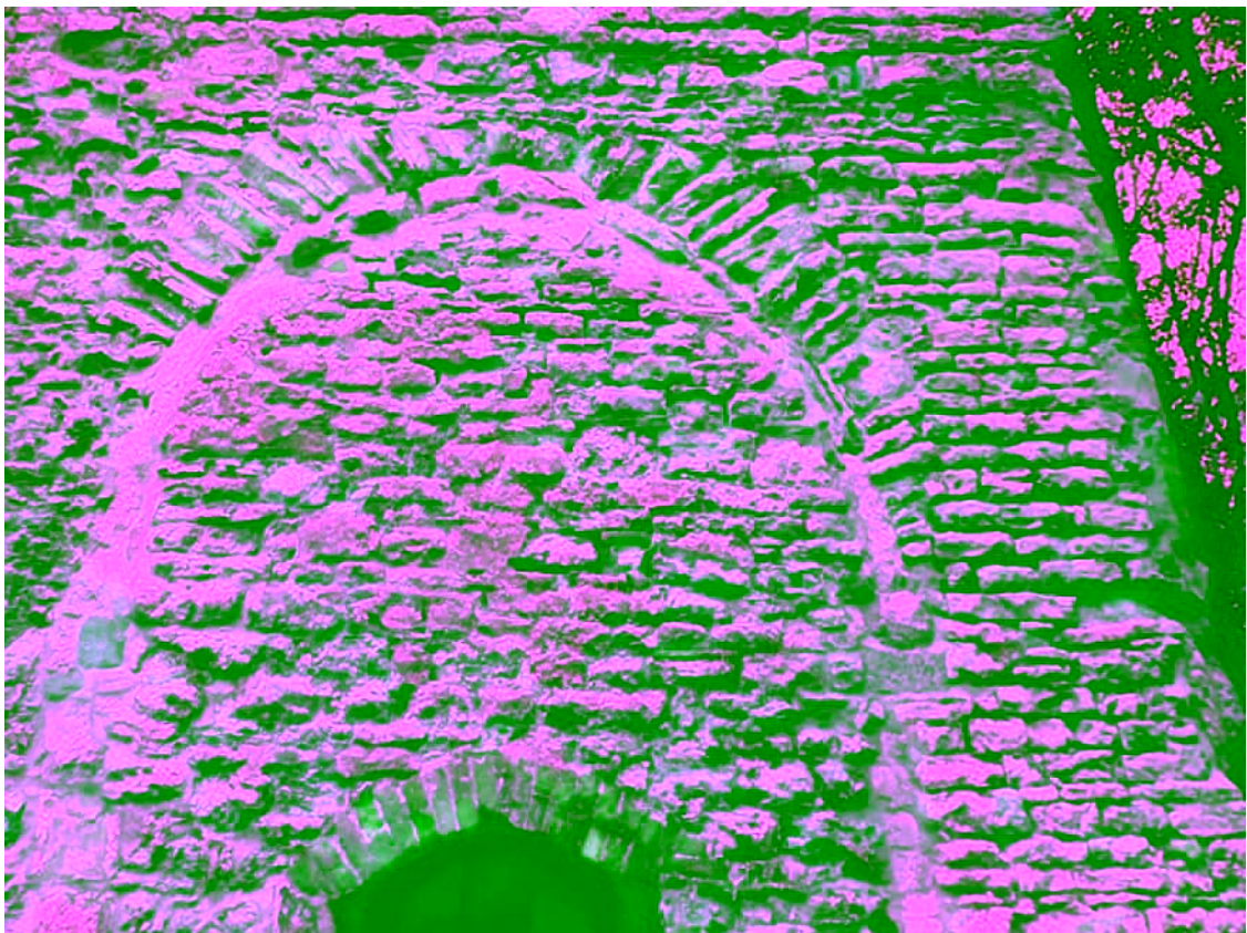
FIGURE 13 St Mary Magdalene: fire-reddened masonry on the S tower arch (photo: the author)
