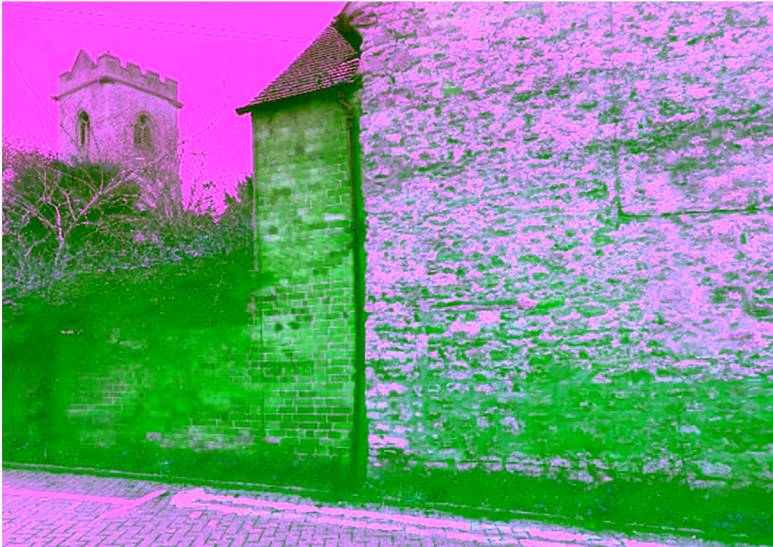
FIGURE 15 No 106 High Street: N elevation showing fire-affected masonry, with St Mary Magdalene tower in the background (photo: the author)
